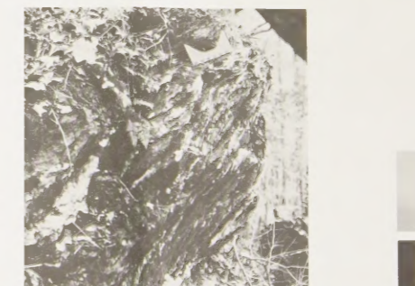
Figure 11. The north-south of the three outcrops at location V13 (P1.1) exposes a 3 ft. thick zone of sericite phyllonite and milky vein quartz. The zone between the outcrops is strongly foliated and bounded by mylonitic gneiss. The contact between the phyllonite and phyllonite is traditionally strongly sheared. The zone of gneiss occurs within both the sericite phyllonite and the main quartz. It is apparent that the gneiss along this contact is strongly schistosity. This zone is indicative of extensive alteration of the gneiss due to the intrusion of hydrothermal, silica-rich fluids into the fault zone, at some time during its evolution. Board is 15 cm long.
